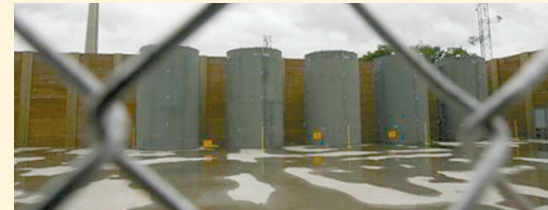
Dry-cask storage at Vermont Yankee
